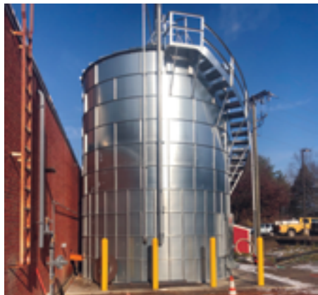
EEI worked with the design team to incorporate a dry wood chip-fired system from Froling Energy of Keene, NH supplemented by in-room heat pumps for Maplewood Nursing Home in Westmoreland, New Hampshire. (Courtesy image)
