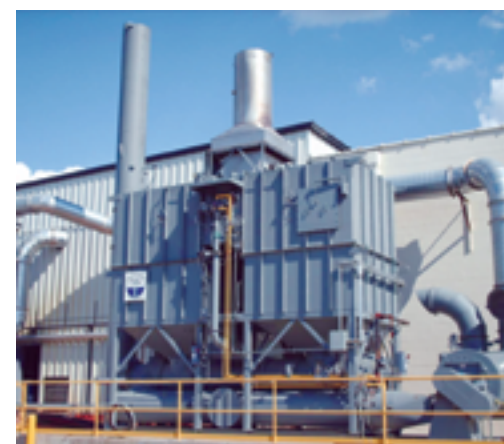
The 10,000 SCFM Ship & Shore Environmental Regenerative Thermal Oxidizer (RTO). (Courtesy photo).
