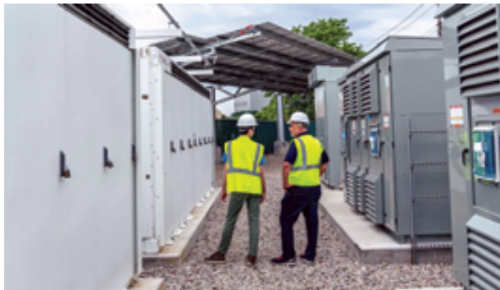
Inside the community battery project built by NineDot Energy in the Pelham Gardens neighborhood of the Bronx in New York City. (NineDot Energy)
