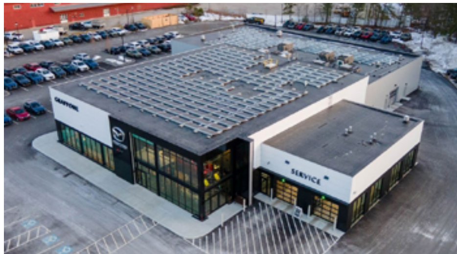
Grappone Mazda with its rooftop solar system installed by ReVision Energy. The 295 solar panels will generate over 160,000 kWh of electricity a year, offsetting more than 60% of their usage. (ReVision Energy)
