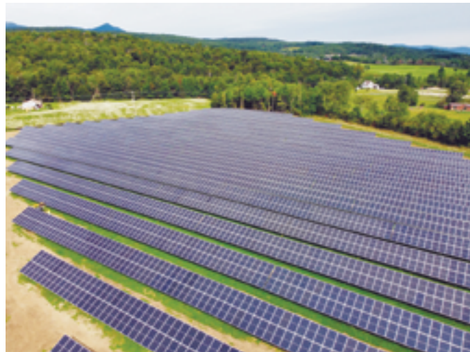
The 2.2 MW Lawrence Brook Solar project is providing low-cost renewable energy to Morrisville Water and Light customers. (Encore Renewable Energy)
