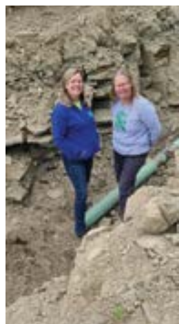
Mulyca Sisters standing in the trench for the new snow making system pipes. General Manager, Marilyn Peterson, is on the left and Carolyn LaHart, Mountain Manager, is on the right.
