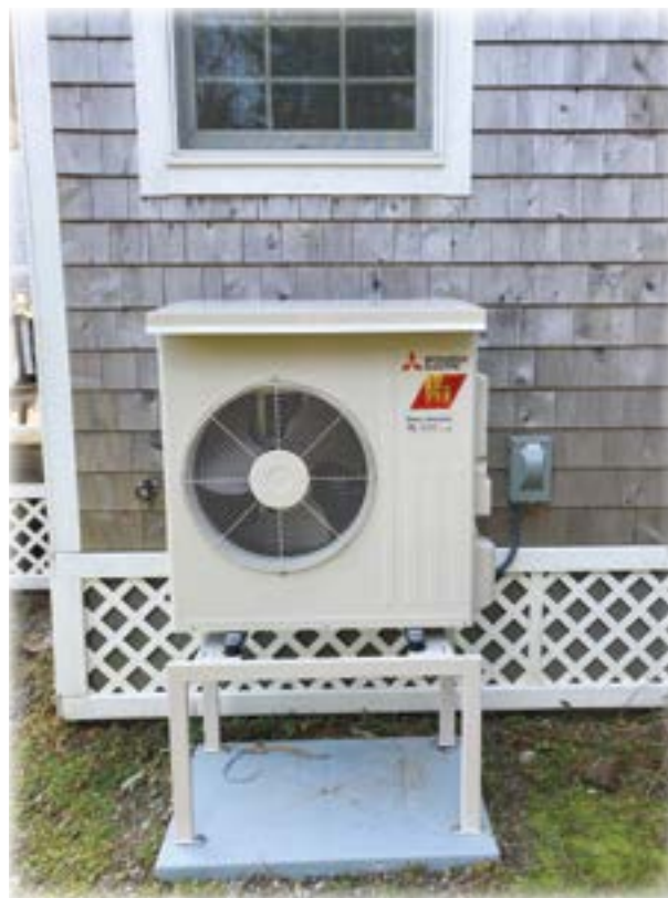
A heat pump installed at the author's house is part of a bulk purchase agreement program. This program is lead by community members to help in reducing their carbon footprint. (Courtesy photo)
