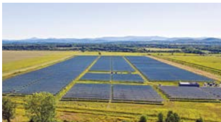
The Panton, VT system is the first U.S. utility-built community microgrid able to run on renewable energy without a fossil-fuel backup. (GMP)
