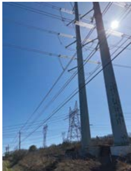
New transmission lines are replacing the old infrastructure all over the capital region of New York State. Shown are old and new lines that cross New Scotland South Rd, near Delmar, NY. (N.R. Mallery)
