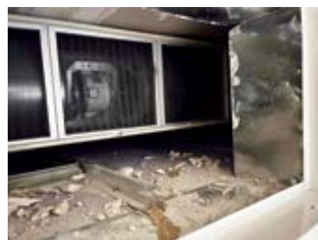
Squeezing a heat pump into a ceiling cavity (top) almost always leads to construction sequencing issues and poor installation. A heat pump without a ducted return allows dust and debris into the system. (Courtesy photo)
