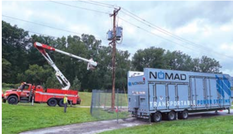
Nomad Transportable Power System on a job site. (Courtesy photo)
