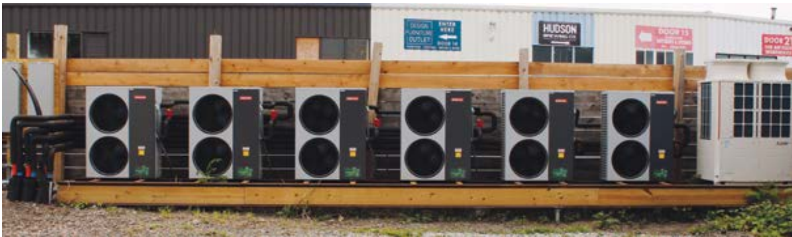
A battery of air-to-water heat pumps provides heats and cools an 18,000 square foot concrete slab of the Basilica Hudson, a popular venue for performances and events in Hudson, New York. The Basilica (on the right) will meet all of their energy needs this year with clean HVAC technologies powered by an on-site solar-photovoltaic system. (Courtesy photos)
