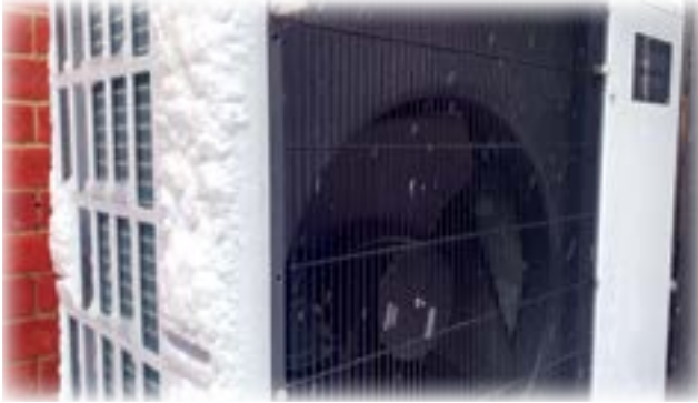
The outdoor unit of an air source heat pump operating in freezing conditions. (Wikipedia)
