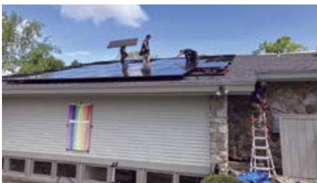
ReVision Energy's crew installing solar on St. Andrew's Church roof. (Courtesy image)
