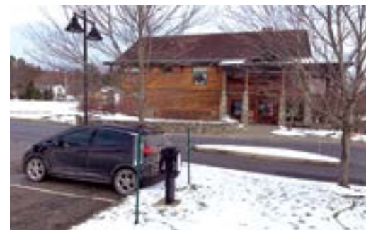
Norwich EV charger installation at Orvis in Manchester, Vermont through the Green Mountain Power Workplace Charger Program. (Courtesy photo).
