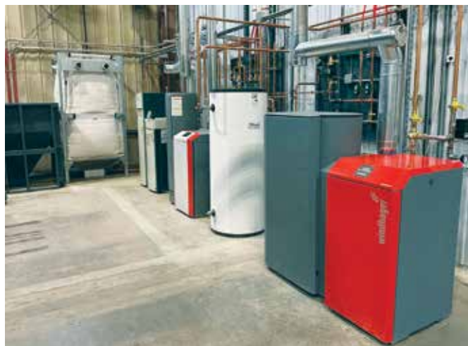
Pellerger's training and demonstration facility in Montpelier, VT houses multiple models of the Windhager pellet boiler and bulk wood pellet storage solutions. (Courtesy image)
