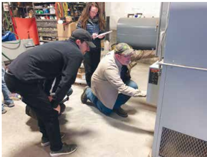
Vermont Tech Renewable Energy student Liam Henchey with Tori Hellwig from the Lamoille County Planning Commission and Nate Brigham from the Village of Johnson collecting nameplate and other information about the buildings' systems during a site visit in March 2023. (Courtesy images)
