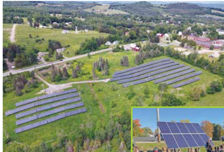
An aerial view of a 500kW AC array in Danville, VT that serves the Caledonia Central Supervisory Union. Inset: Norwich Technologies also installed a small educational solar array at the Danville School to show the students how solar works. (Norwich Technologies)
