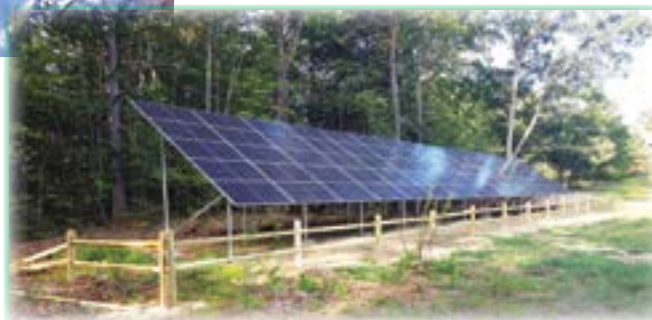
The Starr King solar array in Plymouth, NH. (Images courtesy of NECSS)
