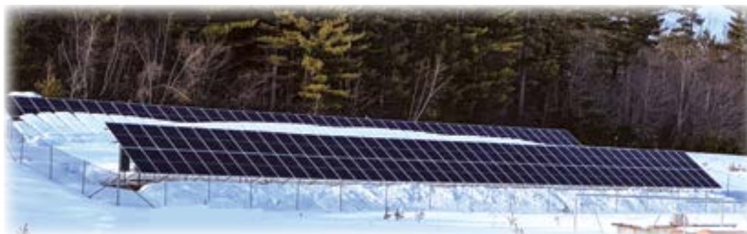
This 63 (DC) kWh array is ground-mounted at an optimum 35-degree angle facing due south on a south-facing slope behind the town ballfield. ReVision Energy installed the solar system. Since monitoring began June 9, 2020, this system has generated 199,115 kilowatt hours of clean energy, offsetting 267,000 pounds of CO2 emissions, and the equivalent of 6784 days of electricity usage in an average American house.
