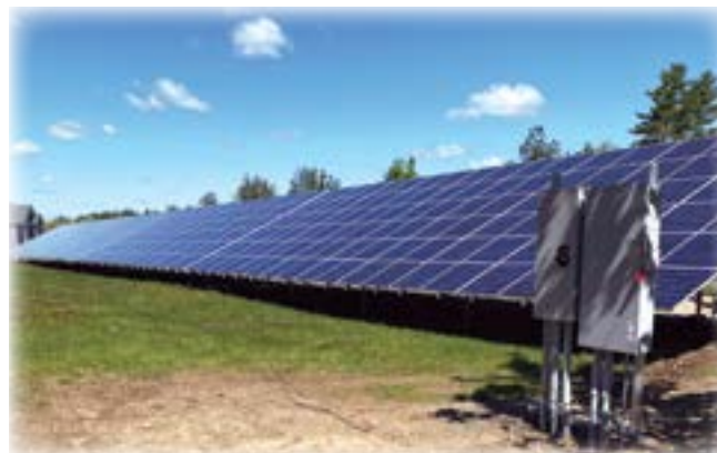
This ground-mount solar array, built in May 2021, is making energy users energy owners. (Courtesy photo)
