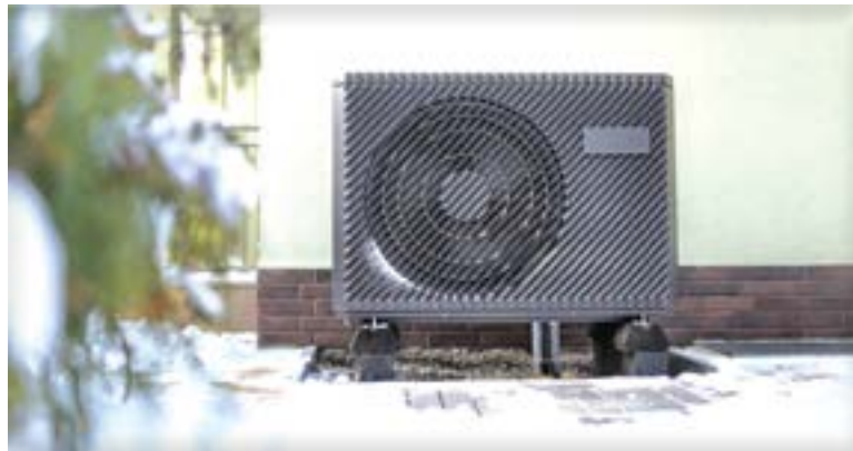
New technologies have increased heat pump effectiveness and efficiency providing benefits to cold-climate residents, and they can now operate with outdoor temperatures as low as -15°F. (tristate.coop)
