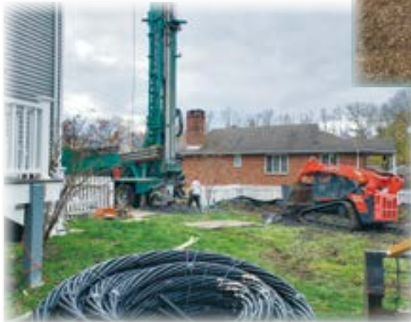
350 ft vertical geothermal heat exchanger being installed by Energy Catalyst. (Images courtesy of Energy Catalyst)
