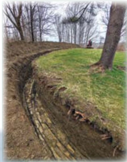
Above: Horizontal geothermal heat exchanger installation in progress. Energy Catalyst offers design and installation of an accompanying geothermal heat exchanger with their heat pumps.
