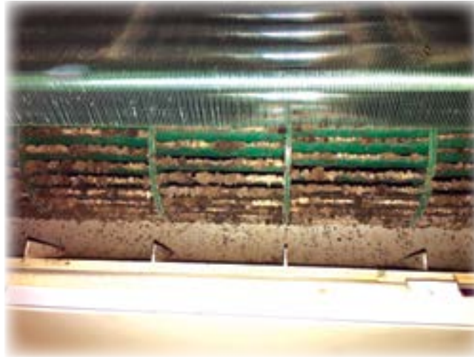
Dirty coils in an air-handler can cause the formation of mold. This also reduces operation efficiency. (Fresh Air Solutions)
