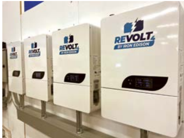
A lineup of four new Iron Edison REVOLT4 batteries. (Courtesy image: Iron Edison)
