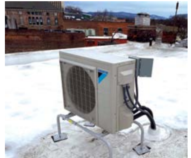
The farm units are heated and cooled by a Daikin two-ton heat pump installed on the roof of the building. (Courtesy photo)
