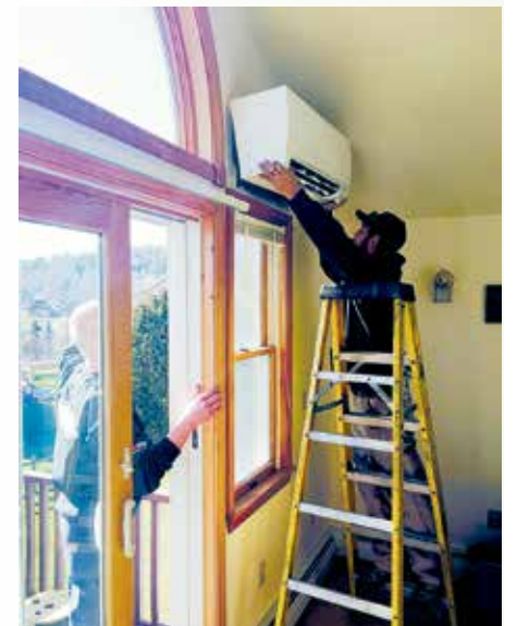
Installing an air-source heat pump will help this homeowner use half the energy needed for propane and oil systems. Photo: Steve Costello, GMP.
