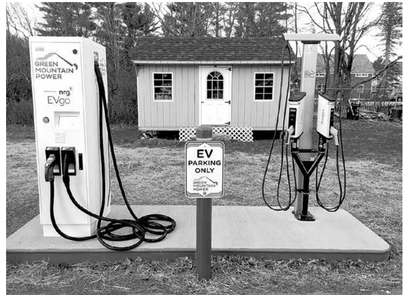
Charging station at Northshire Bookstore. Photo Courtesy of Chris Morrow, Managing Partner
