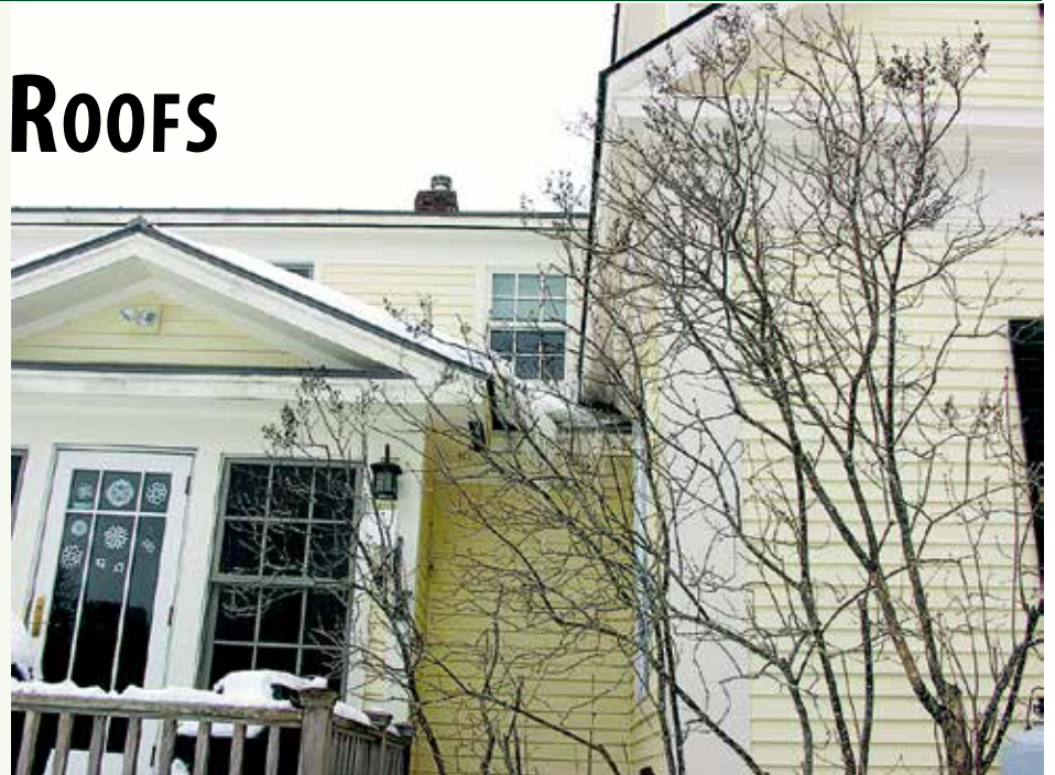
Converging roofs led to snow and ice accumulation which caused interior wall leaks.
