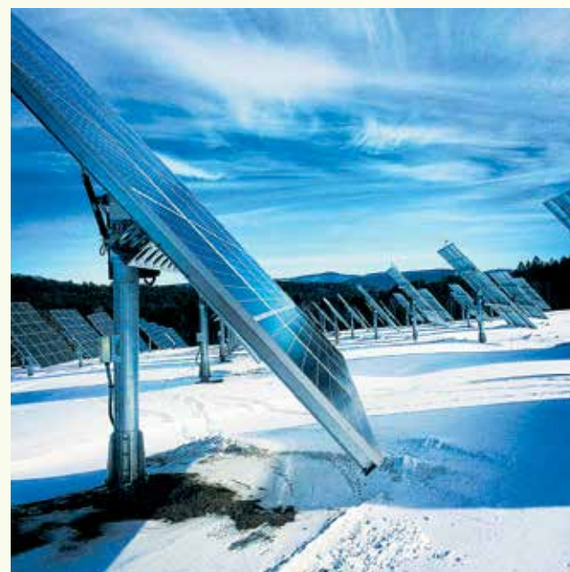
Net-metered PV array. Photo courtesy of All Earth Renewables.
