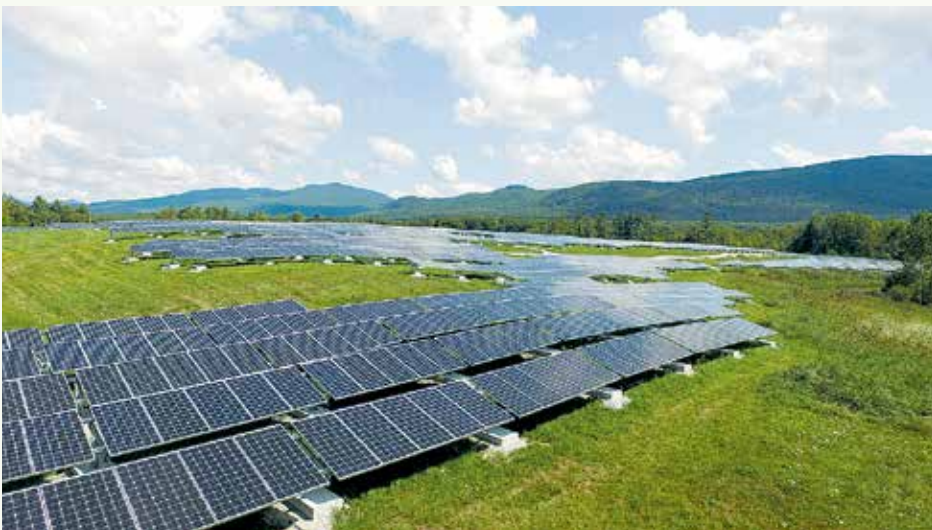
Stafford Hill Solar Farm, Rutland, VT. Photo: Eric Hudiburg.
