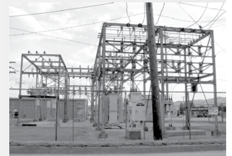
An electrical substation in Roaring Spring, Pennsylvania. Photo by Andrew Bossi CC-BY-SA-2.5
