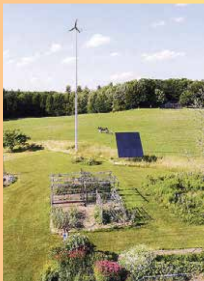
A single inverter works with both solar photovoltaics and wind power this system in Gorham, Maine. Photo courtesy of Pika Energy.
