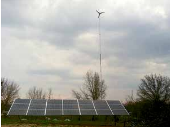
Pika's inverters handle a combination power from different sources, making it easy to demonstrate different kinds of renewable energy to students. Courtesy of Pika Energy.
