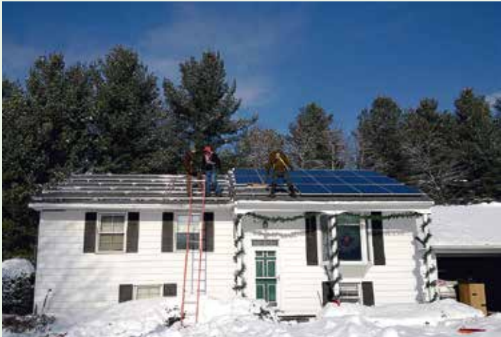
A residential solar installation in Queensbury, NY in the winter of 2014. Photo courtesy of Ben Sopczyk from 'Active Solar.'
