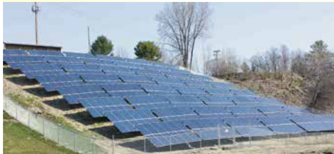
The Cavendish, VT 148kW PV array is truly hidden. Folks in town want to know where it is and how they can see it. Photo courtesy of Peter LaBelle.
