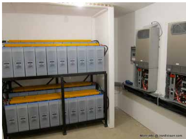
Cadillac, Mi - wind and solar compatible battery. Photo courtesy of Iron Edison.
