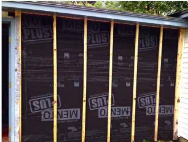
Exterior vapor open membrane with vertical strapping to create a rain screen. Photo by Michael Goetinck.
